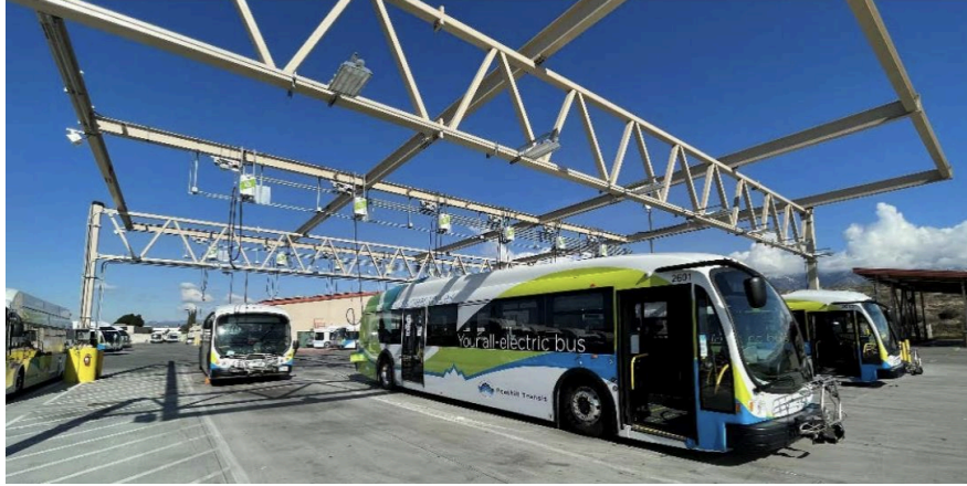
Foothill Transit depot-based overhead pantograph charging
